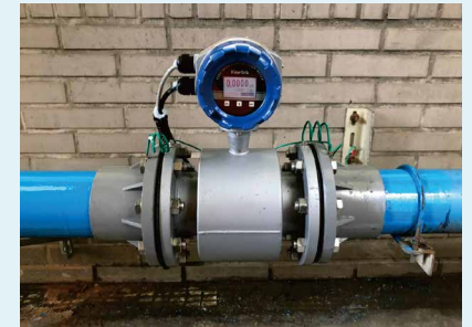
Wastewater flow detection
