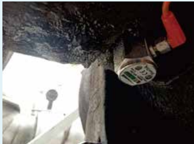
Pipeline flow detection
