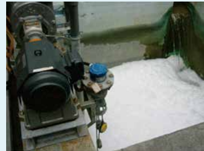
Wastewater level detection
