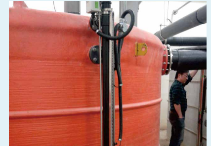
Cooling water reserve detection of electronic plants
